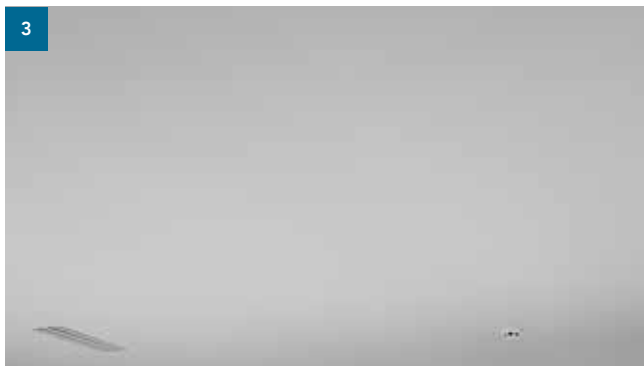
Sanding of dry joints and spraying of the area. Sand the surface around the hole in order to remove the excess render.
