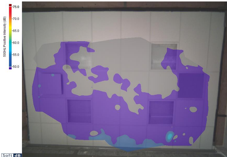
Fig. 5 – A color map showing sound transmission through the ceiling and plenum barrier combination, 500 Hz octave band, stone wool ceiling panels (NRC 0.95, CAC_{panel} 22), double-layer plenum barrier. Using a plenum barrier improved overall performance to CAC_{system} 49.
