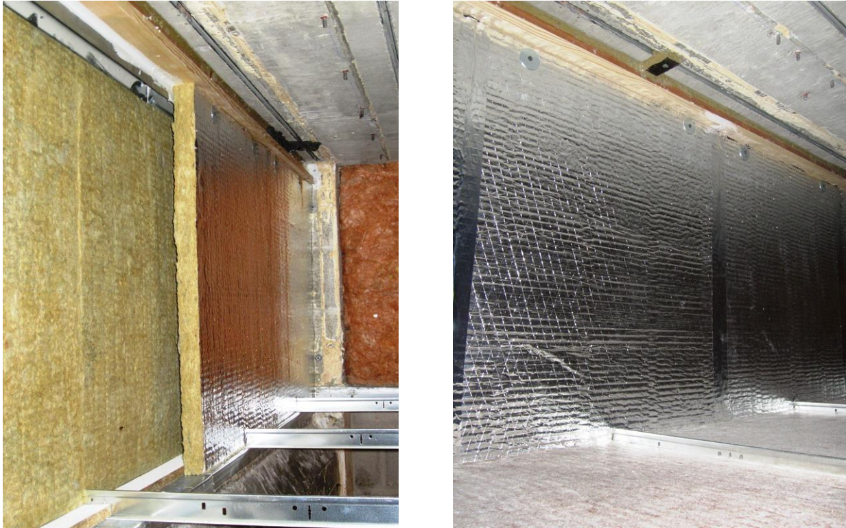
Fig. 2 - Lightweight, stone wool, plenum barriers installed above the central demising wall of the laboratory's chamber during some tests. Top-left: Single-layer. Top-right: Double-layer with a 42 mm (1-5/8 inches) airspace in between. Bottom-left: Double-layer with seams staggered and small cuts at the bottom so the panels slide down over the grid bulb. Bottom-right: Intallation complete with tops screwed, seams taped and ceiling panels installed.
