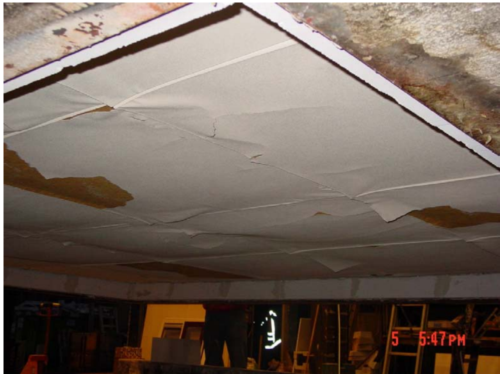
Figure C3 Specimen after the test looking into the cavity
