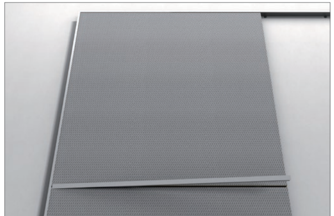
3.6 Cover the horizontal joints between panels by clicking T24 profiles into the T fixing brackets, then slide it carefully under the J-channel edge. These horizontal tees must be cut to an exact dimension of M-12 mm.
