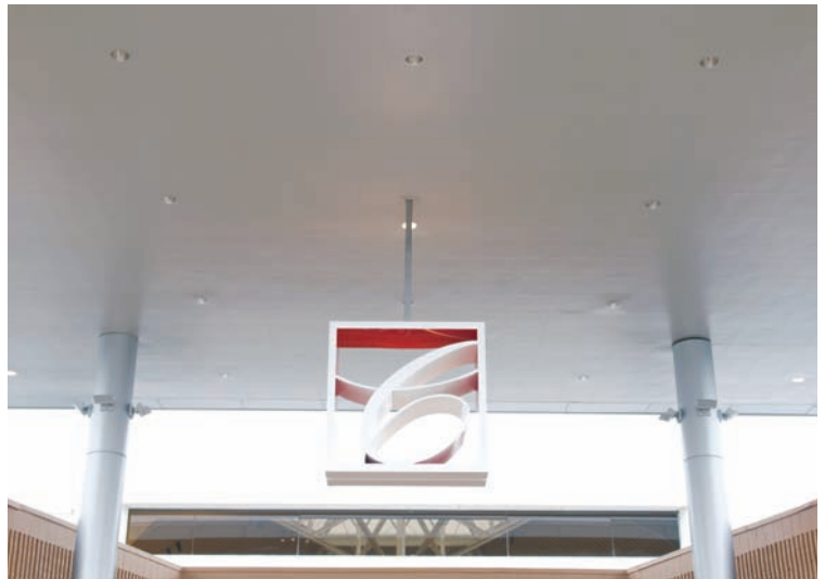
To revitalize Christiana Mall in Newark, Delaware, owners relied on multiple metal ceiling systems. Designed to withstand positive and negative wind pressure and extreme weather, snap-in metal panels were painted in a durable silver finish and installed as soffits under the exterior canopies.
